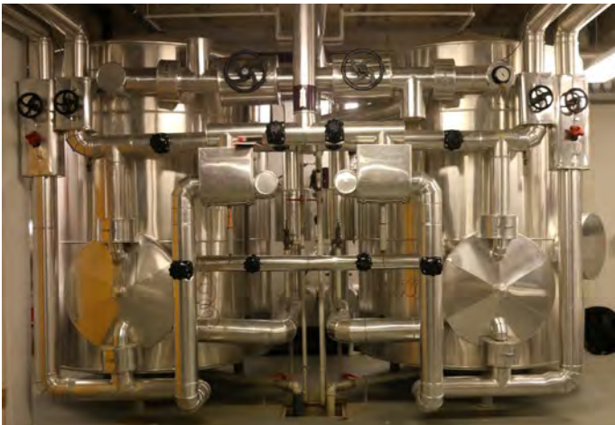
One of the two hot water preparation plants at the regional hospital of Viborg
