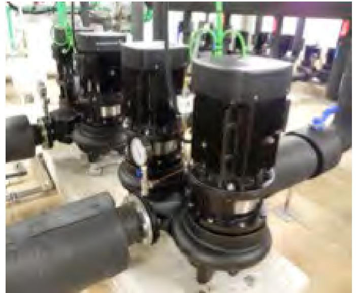
Grundfos TPD twin pumps used in a medium size chilled water plant
