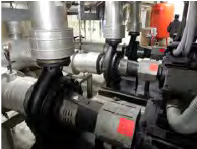
Secondary pumps in a large stadium chilled water plant
